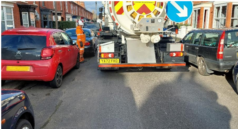
Photograph 2 Gully tanker operation restricted by parked vehicles.
